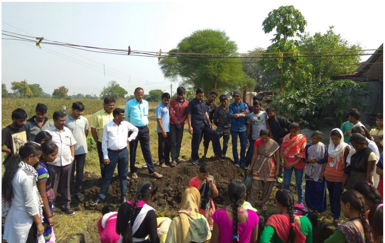
Construction of Soak Pit for Water Harvesting Purpose near Gram Panchayat Bore well. 05/01/2018 during the camp.
