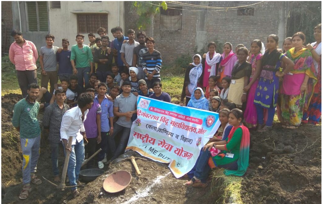
Construction of Soak Pit for Water Harvesting Purpose near Gram Panchayat Bore well. 05/01/2018 during the camp.
