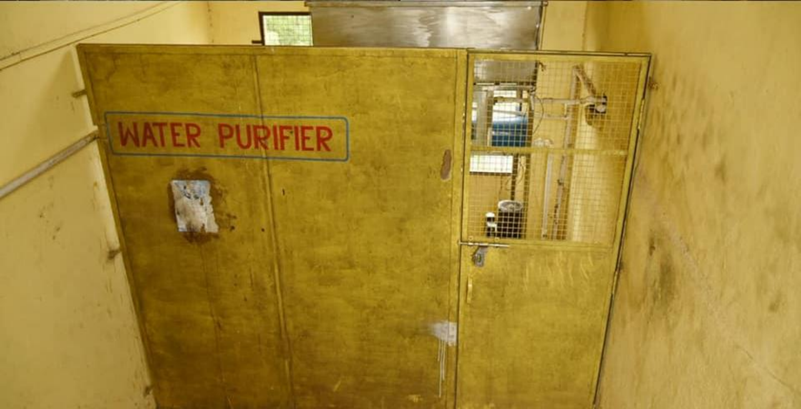
Water Purifier system
