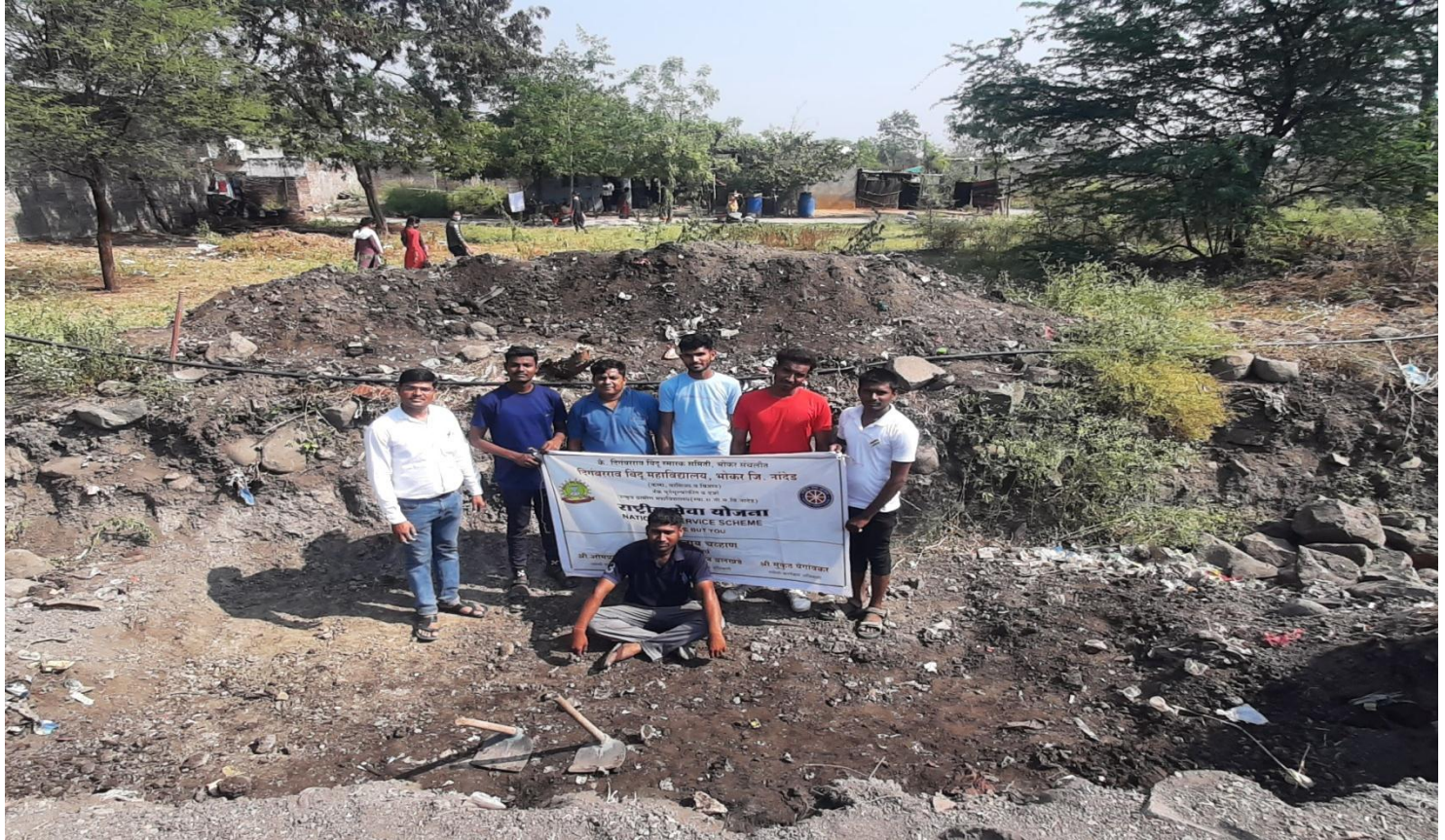
Soak pit for rain water harvesting.
